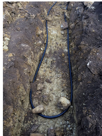
Pipes laid In trench in above installation. 8 trenches were dug in total.
