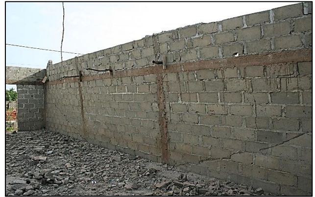
A wall damaged by monsoon weather in the Gambia.
