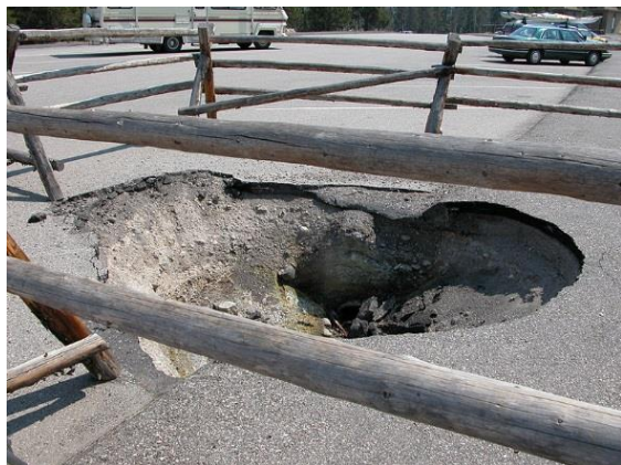
Figure 5. Sink hole in a parking lot at Yellowstone National Park, USA.
