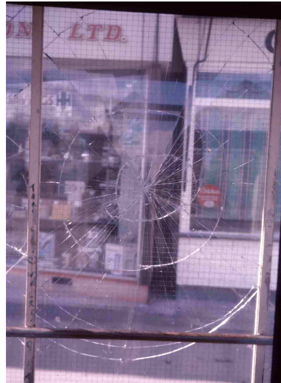
Fracture patterns in wired glass in a bus shelter after a brick had been thrown at it. (Photograph by Peter Kennett)
